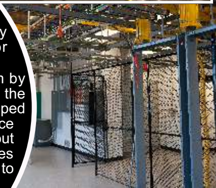
Continuously building telecom sites
